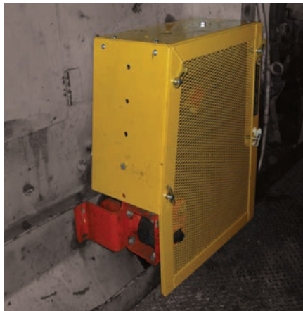
2 Guard installed over exposed conveyor pulley
